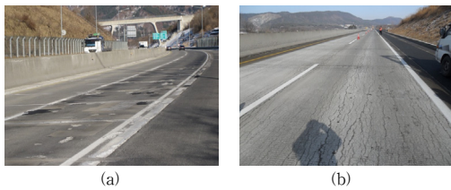
[Fig. 6] Concrete Pavement Deterioration Influenced by Environmental factor
