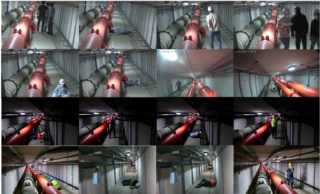
Fig. 1. Sample images of workers in the underground utility tunnel
