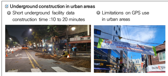
Fig. 1. Limitations of constructing underground facility data during underground construction of communication lines in the air
