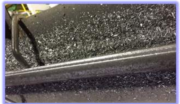
(d) Crane derailment due to rail damage
